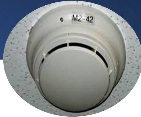
Typical Building Fire Alarm Smoke Detector
